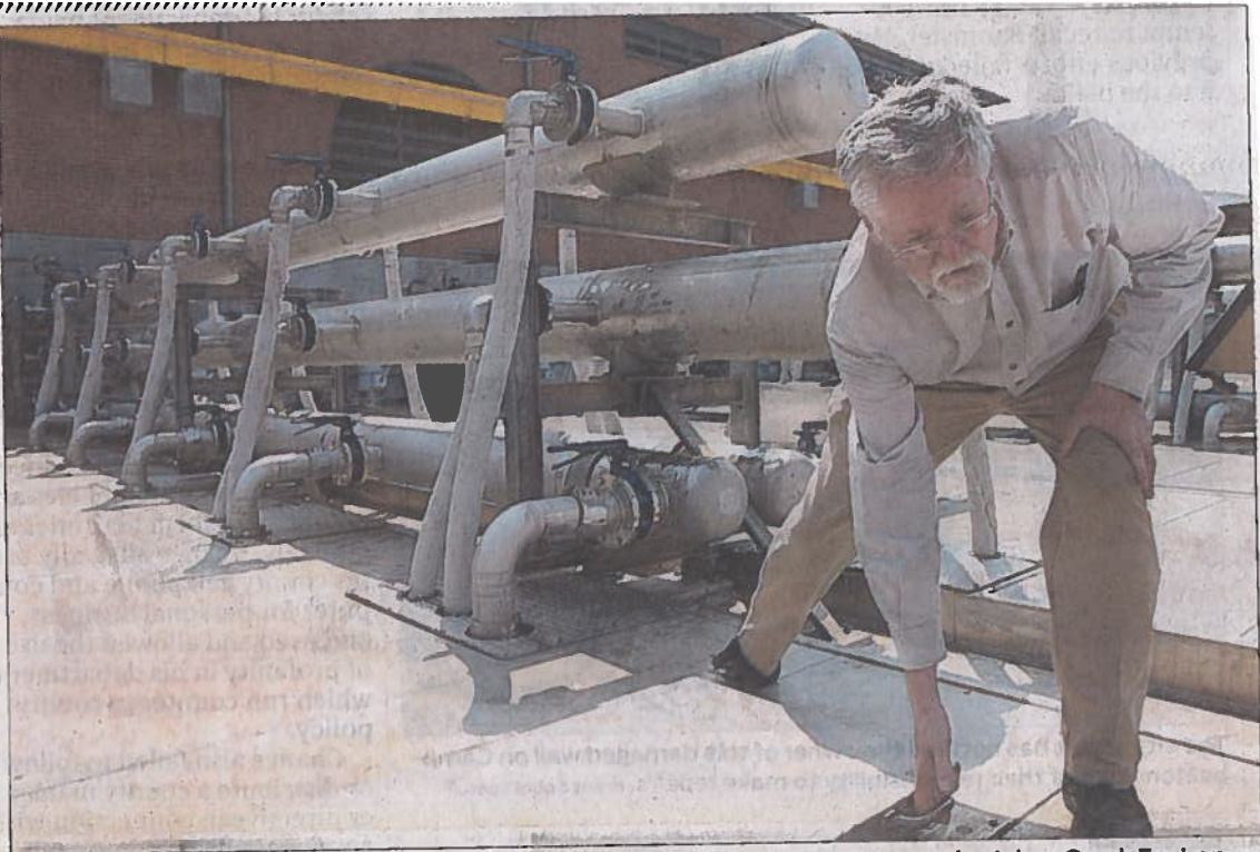
Senior operator William Francis shows the membrane biological reactor area at the Johns Creek Environmental Campus, Fulton County's newest water treatment reclamation plant. Vino Wong vwong@ajc.com
